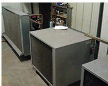
(4) Climate Control cooling units
