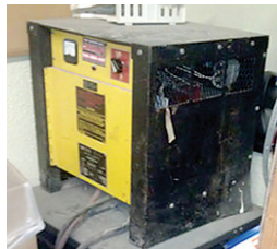
Fork lift charger
